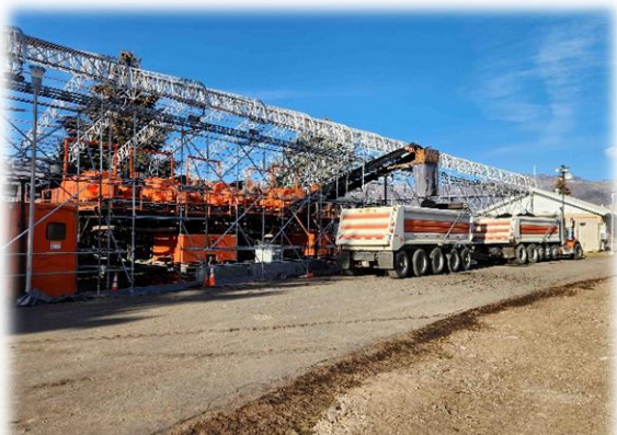
Centrifuges and Conveyors Loading Dewatered Solids into Truck
